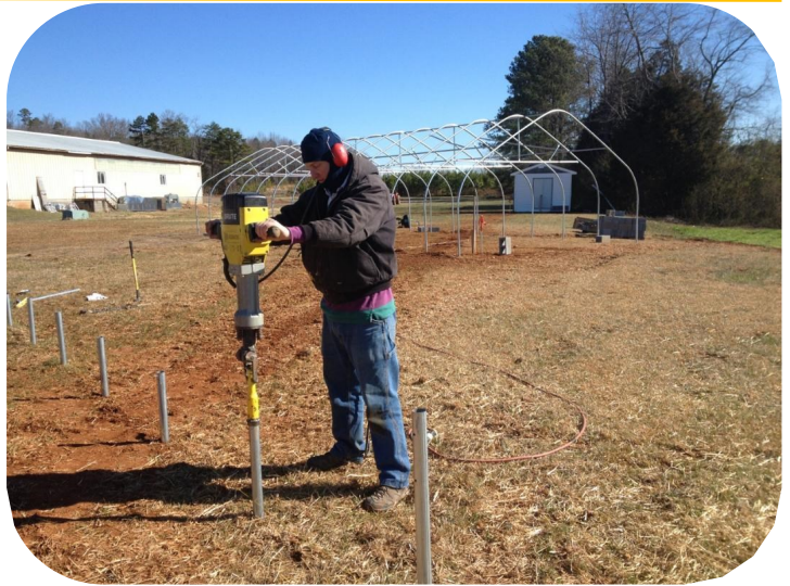
Using an electric jackhammer to sink ground tubes. Published with permission from: George Washington Carver Agricultural Initiative, Culpeper, VA
