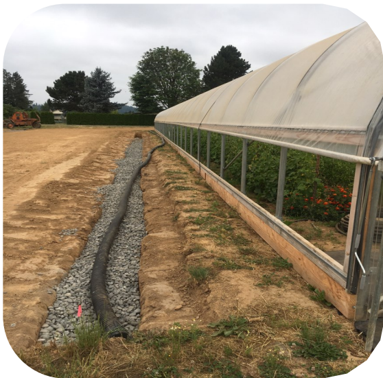
Greenhouse drainage pit.. Published with permission from East Multnomah Soil & Water Conservation District, OR
