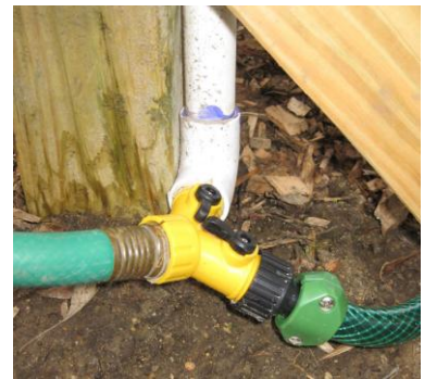
Figure 6. "Y" splitter on supply line
