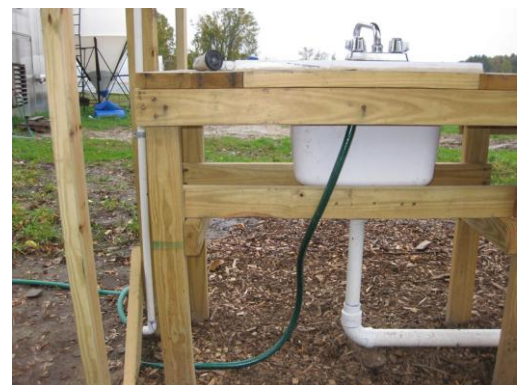
Figure 2. Hand Wash Sink Water Supply
