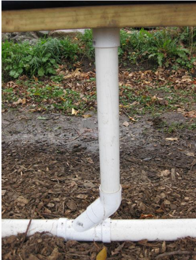
Figure 9. Wash tub drain pipes
