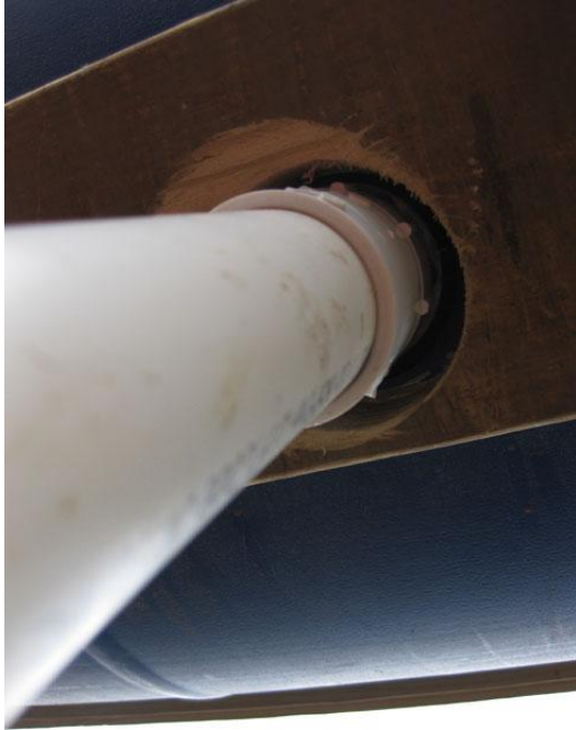
Figure 3. Blue tub drainage
